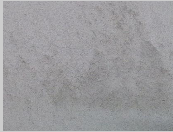
after being cleaned with mould stain remover
