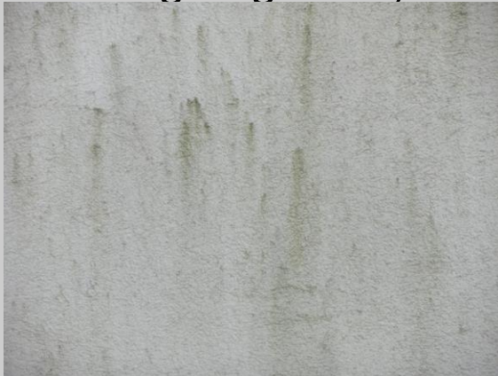
Algae growth on silicate plaster
